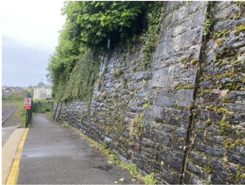
Figure 5: End of existing platform where extension can commence (start of fence) – careful consideration of interface with existing retaining wall necessary
